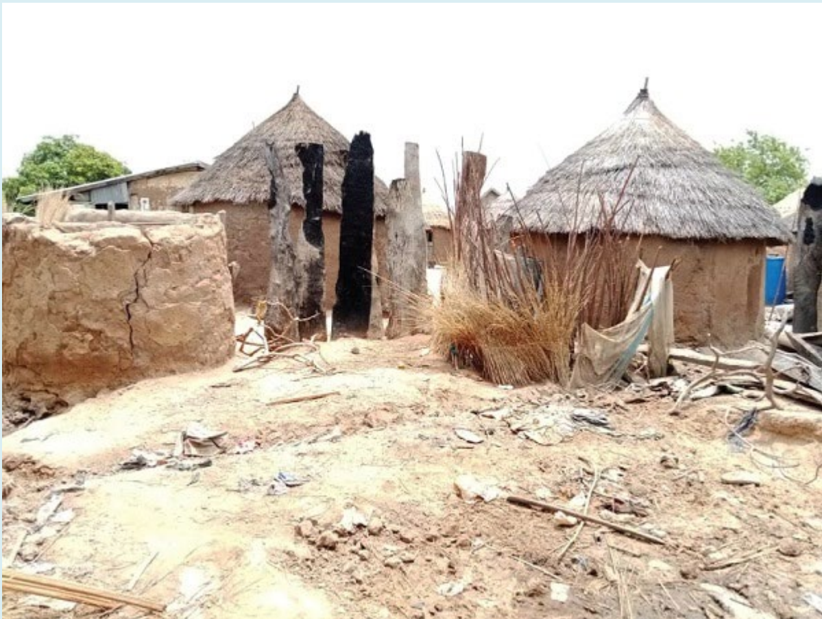
Remains of some buildings that were torched during the communal clash (arrowed)
